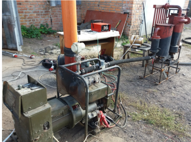
Fig. 1. Exterior of experimental plant
